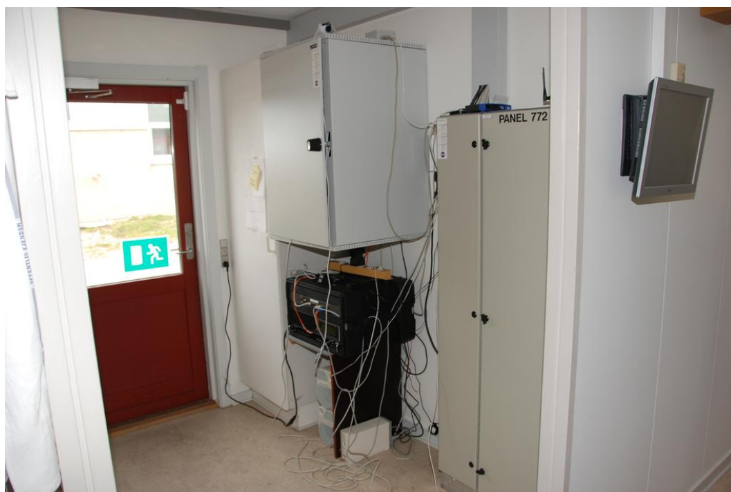
Figure B.7: The server hardware.
